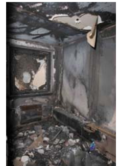
The ferocious fire blew out the window and destroyed almost everything inside the bedroom
