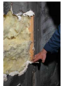
Burned plasterboard is ripped away to show no damage to the timber frame structure at all
